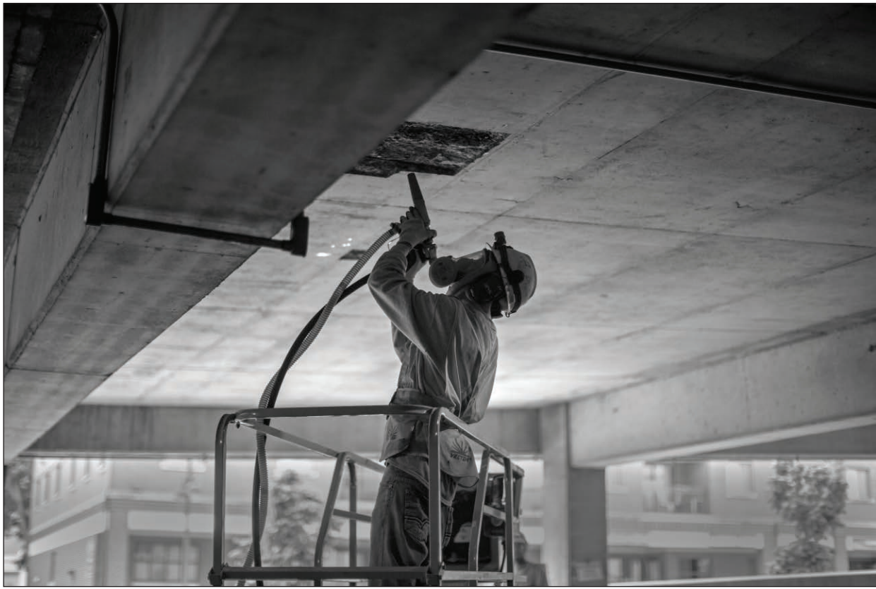
A construction worker clears out dust from a recently open space in the Dubuque Street parking ramp on Wednesday. Construction has shut down most of the lower levels in the ramp. (The Daily Iowan/Sergio Flores)
