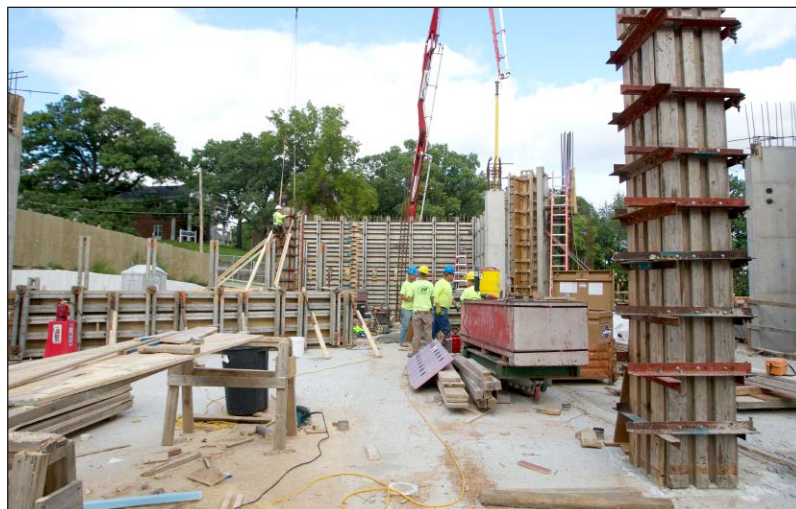
Construction workers continue to build the Art Building replacement near River Street on Sept. 11. The building is scheduled for completion in May 2016. (The Daily Iowan/Valerie Burke)
