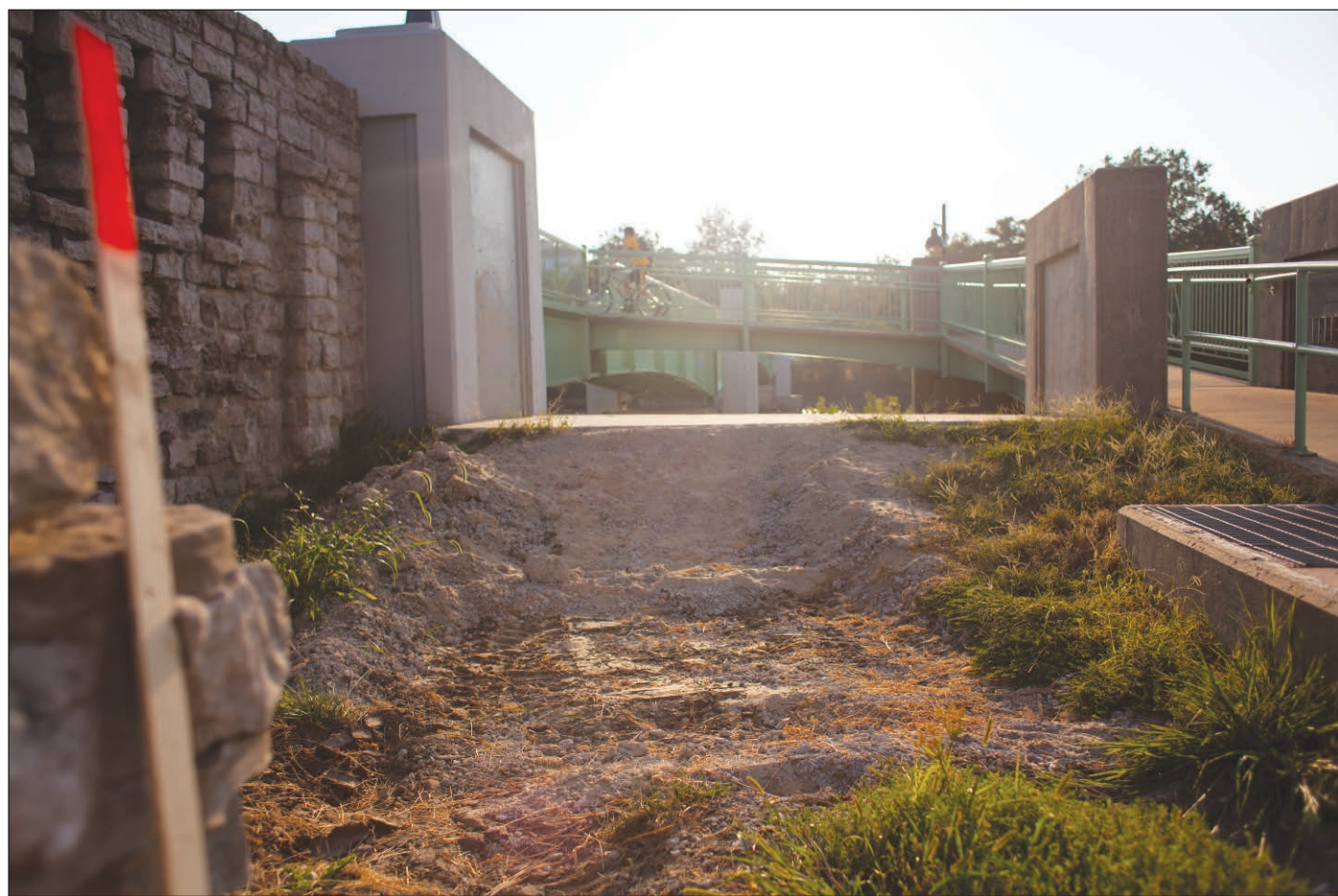
The area around the pedestrian bridge near the IMU is damaged after the flood on May 31. The floodwaters caused damage to the landscape in areas of campus. (The Daily Iowan/Joshua Housing)
