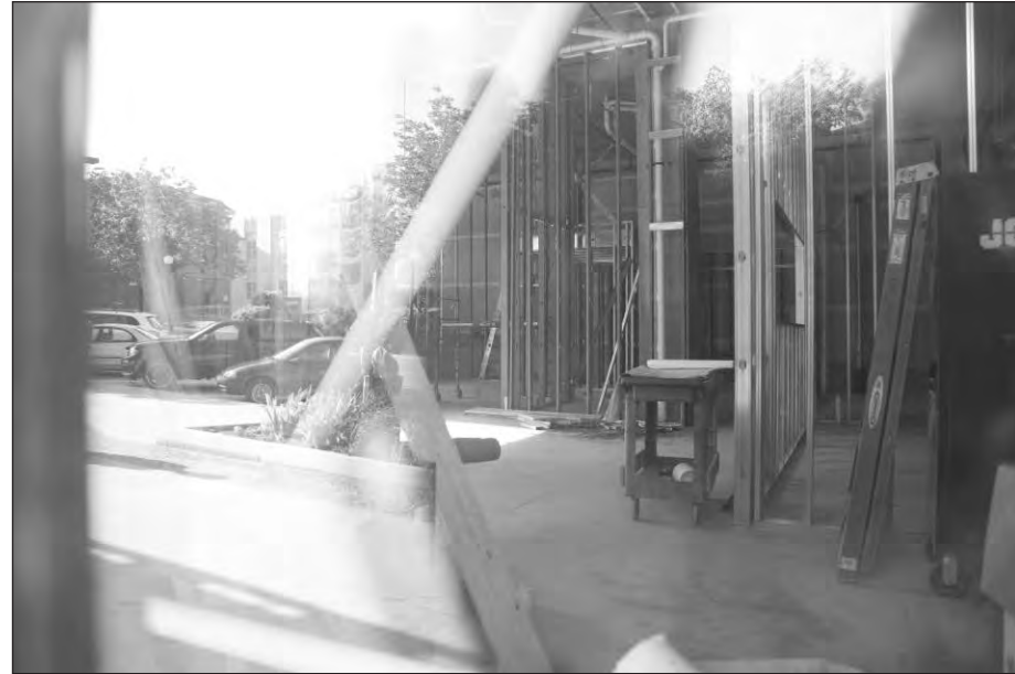
Construction has started on Teddy's Bigger Burgers on East Washington Street, as seen on Monday. Teddy's is a Hawaii-based burger restaurant. (The Daily Iowan/Callie Mitchell)
