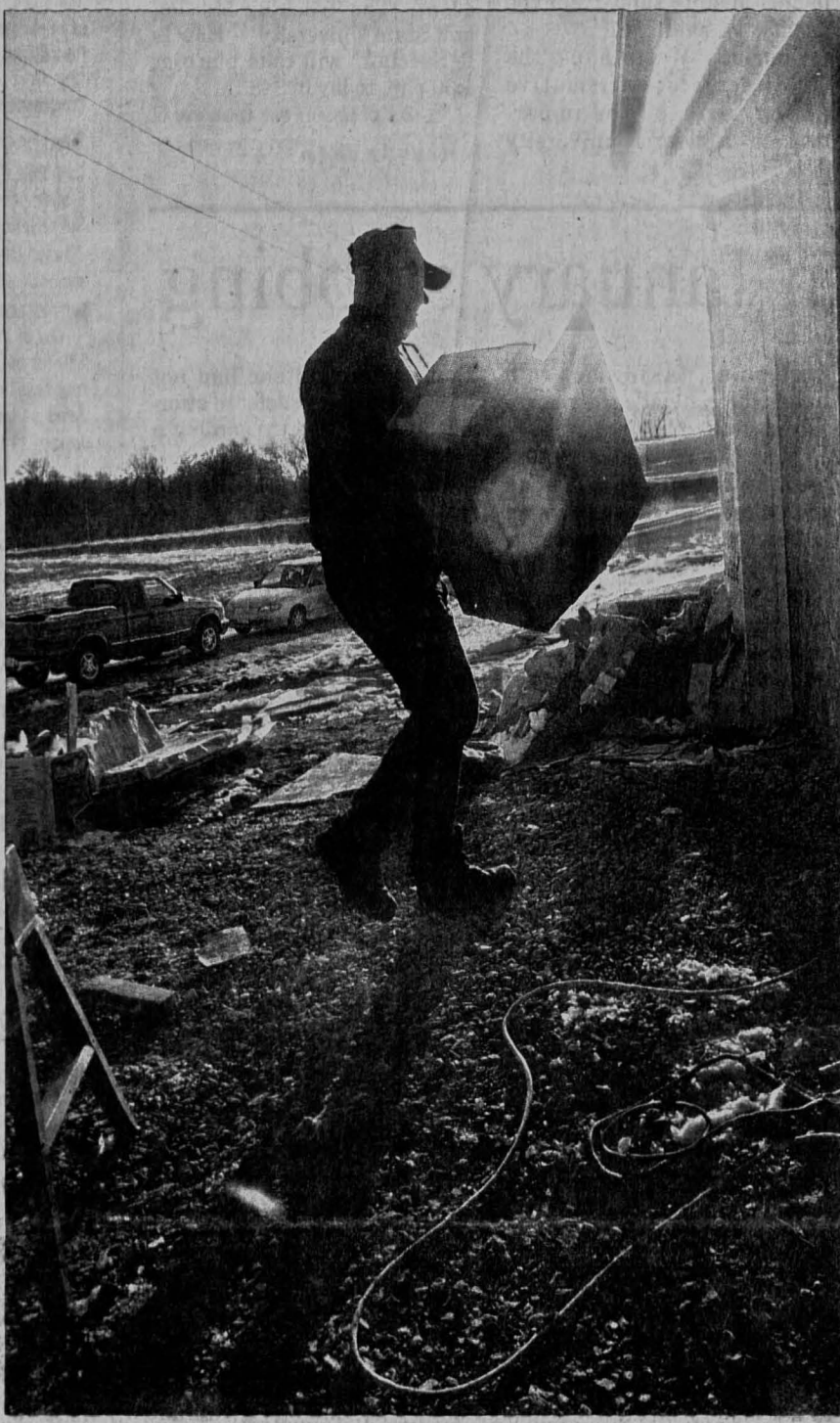
Whitney Kidder/The Daily Iowan Bruce Timmins, a Gulf War veteran, carries a box into the house his construction company is building just outside of Washington, Iowa.
