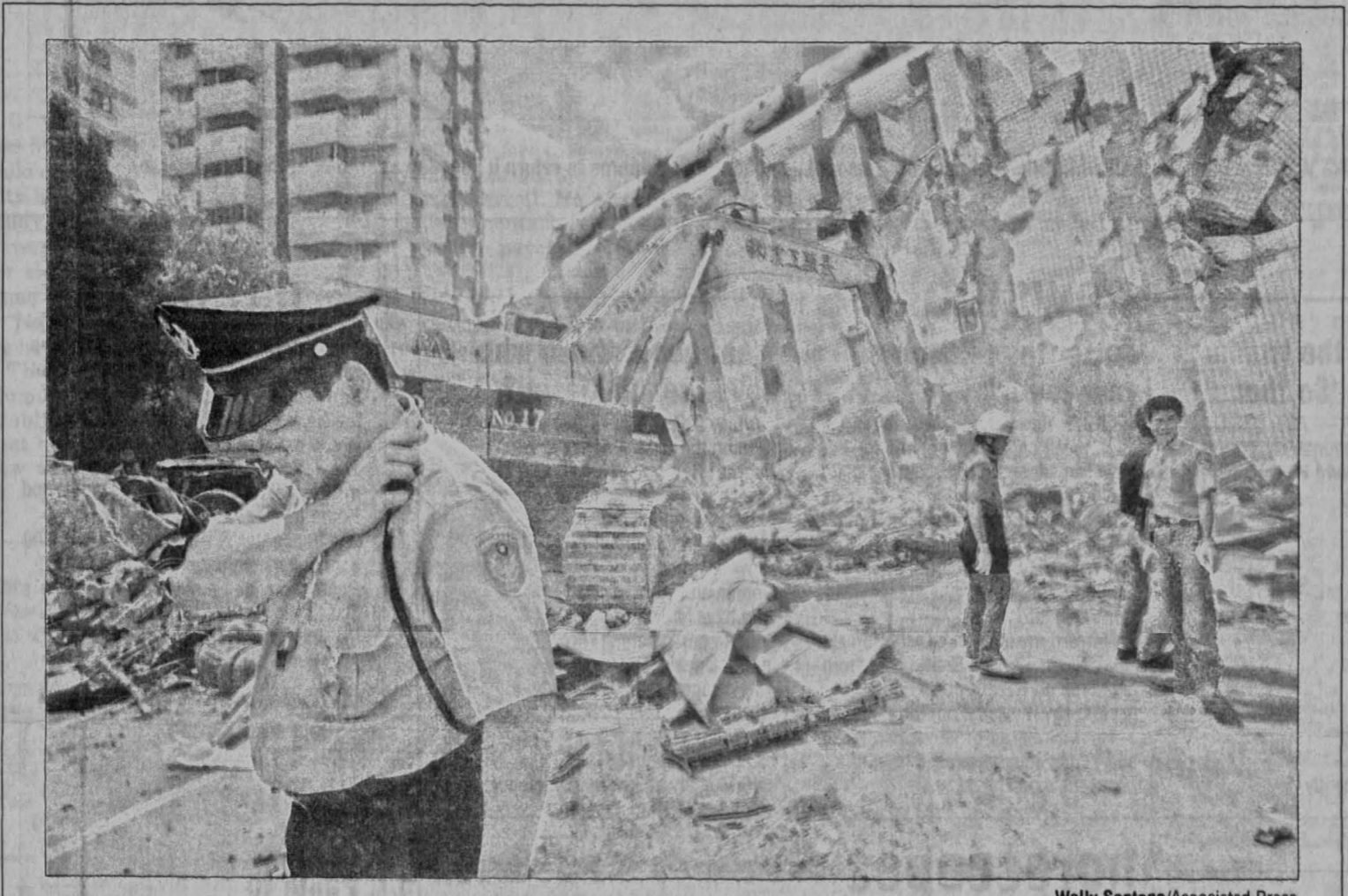
A police officer listens to his radio in Fengyuan, Taiwan, as workers demolish a collapsed building after an earthquake Tuesday.
