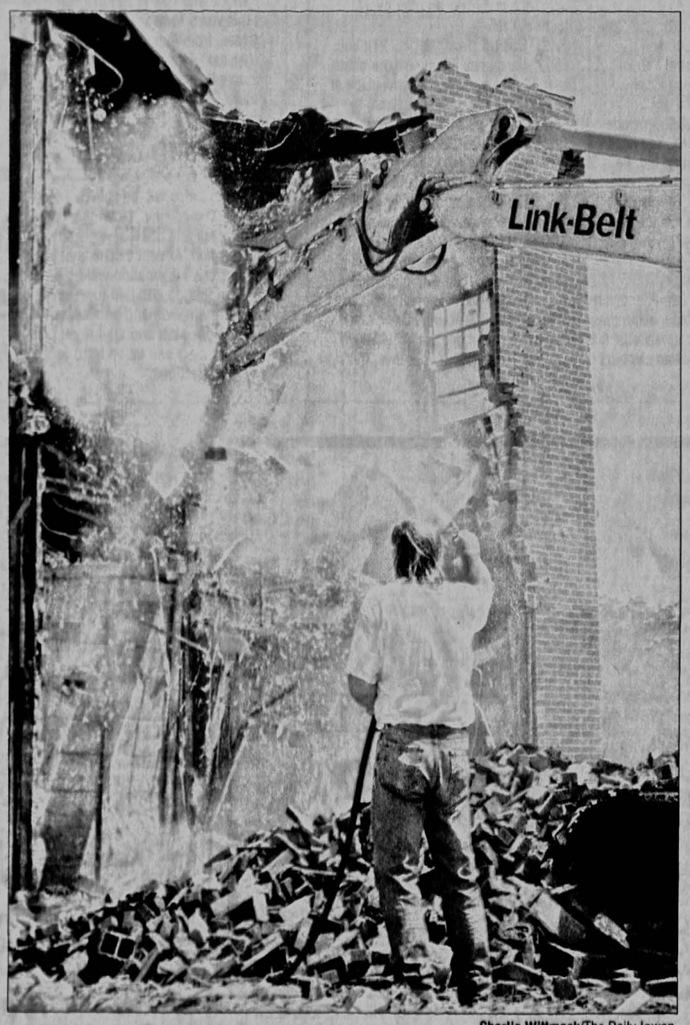
Demolition of the Harmon Building, 2 S. Linn St., began Wednesday to make way for a parking ramp at the site. Many residents had hoped to save the building by making it an Iowa City historic landmark. Charlie Wittmack/The Daily Iowan
