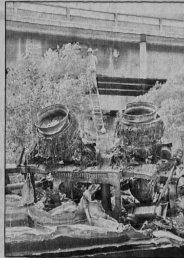
Jerry James Hynes Jr./The Daily Iowan Members of the Iowa Department of Transportation bridge inspection team examine the fire damage after an accident Wednesday on I-80.
