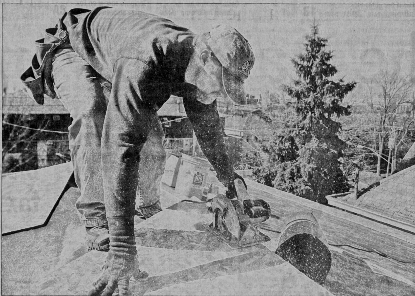
Vance Duve cuts a piece of plywood to fit the corner of a roof on an apartment building in the 400 block of South Johnson Street Monday afternoon. Duve is on a crew re-shingling the roof. Above average temperatures have accelerated area construction projects, and he expects to be done by Thursday.
