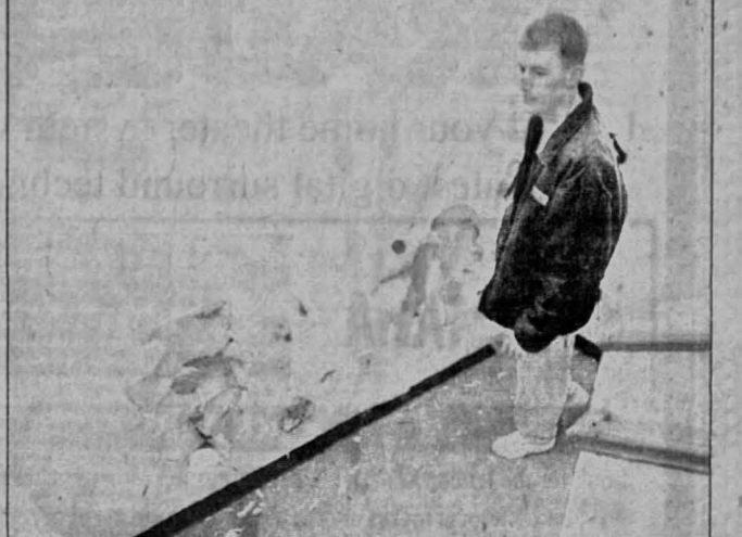
Brian Ray/The Daily Iowan UI sophomore Dyson Miguel walks up a damaged stairwell in the Kennedy Center apartment complex Monday. "It bothers me that this happens," Miguel said.
