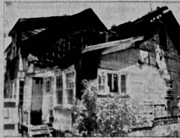
The house at 901 Walnut St. caught fire early Wednesday morning in what officials are suspecting as arson.
