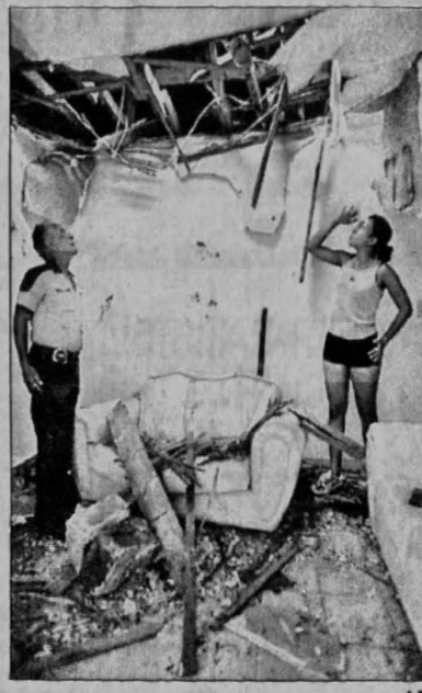
Orlando Rodriguez looks up at the hole in the roof of Younet Fumero's apartment a tornado touched down in Miami on Monday.
