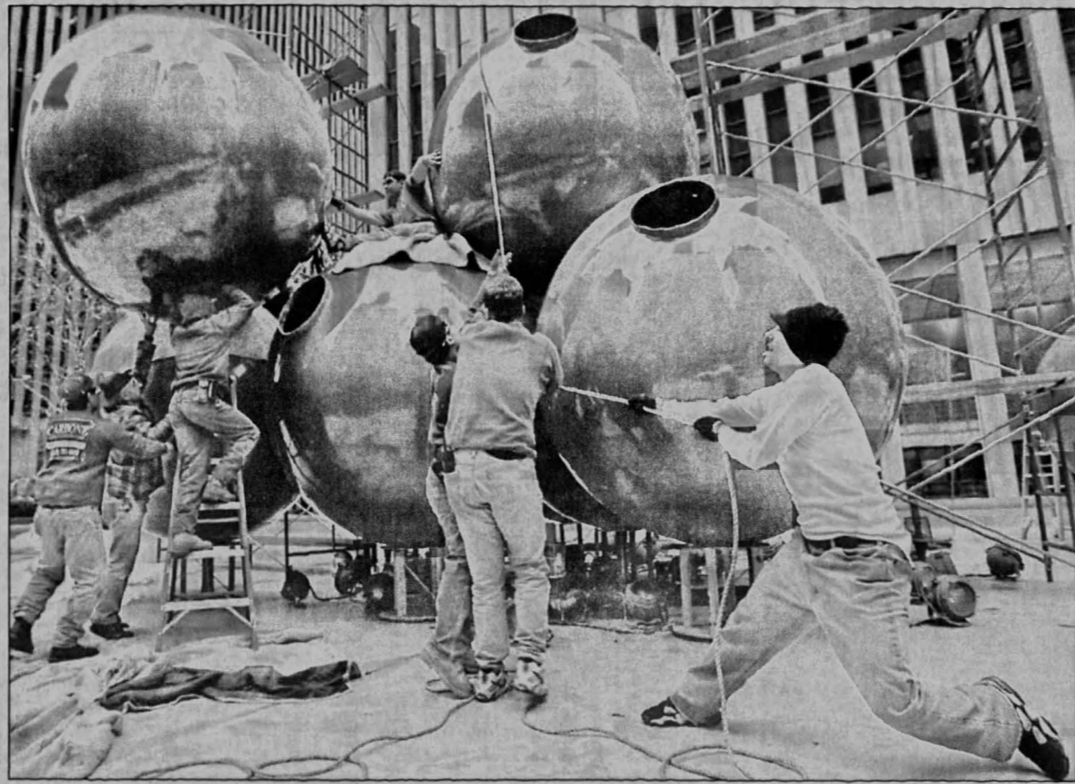
Workers from Cardone Improvements hoist ornaments outside of an office building in midtown Manhattan Monday.
