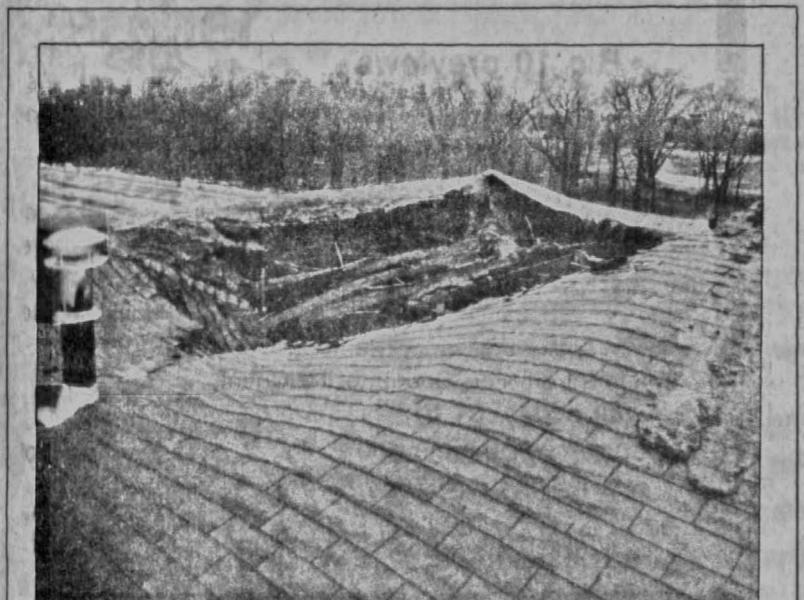
The roof of an apartment building located at 1910 S. Gilbert St. shows the charred hole resulting from a fire early Friday morning. The cause of the blaze is still under investigation by the Iowa City Fire Department.
