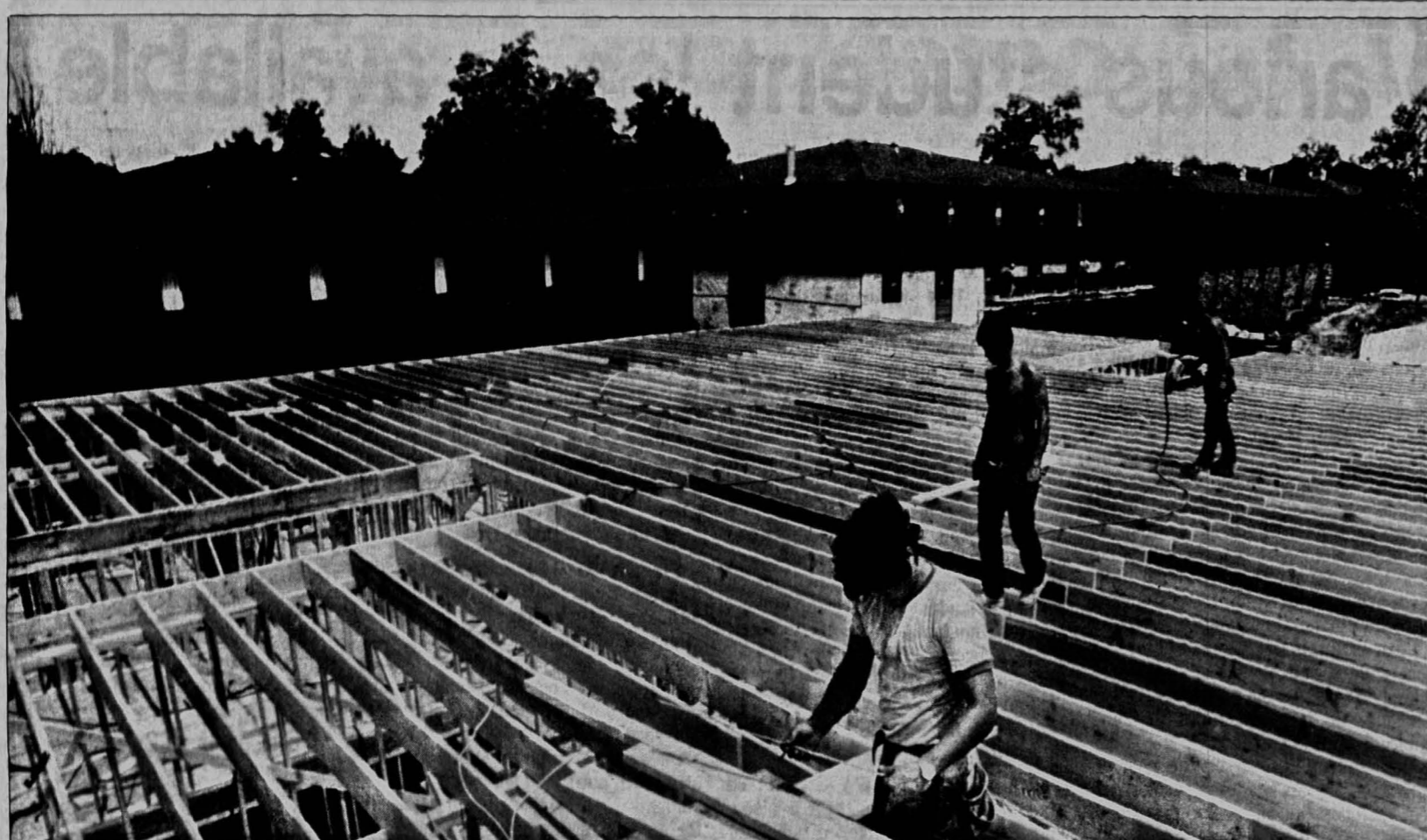
Construction laborers work on putting up one of several new apartment buildings on South Van Buren Street.
