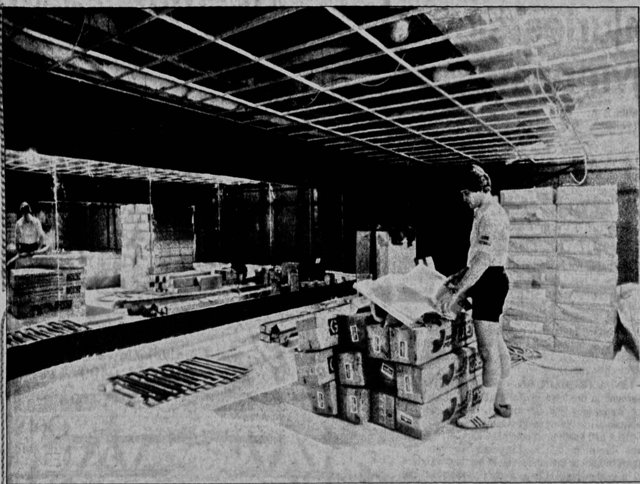
Iowa strength Coach Bill Dervrich scrutinizes the blueprints of the new weight lifting room connected to the Recreation Building. The new structure is due to be completed March 1 and will be used for training and instruction.
