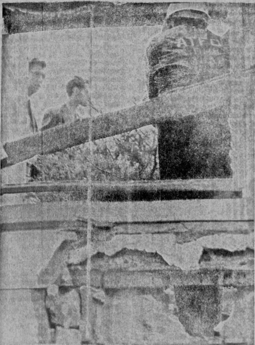
A federal agent from the U.S. Treasury Department's Alcohol, Tobacco and Firearms Division (ATFD) bomb squad checks the area around the Iowa City Civic Center where a bomb exploded early Friday morning. The bomb knocked a large hole in the foundation of the building, shown at the bottom of the picture.
