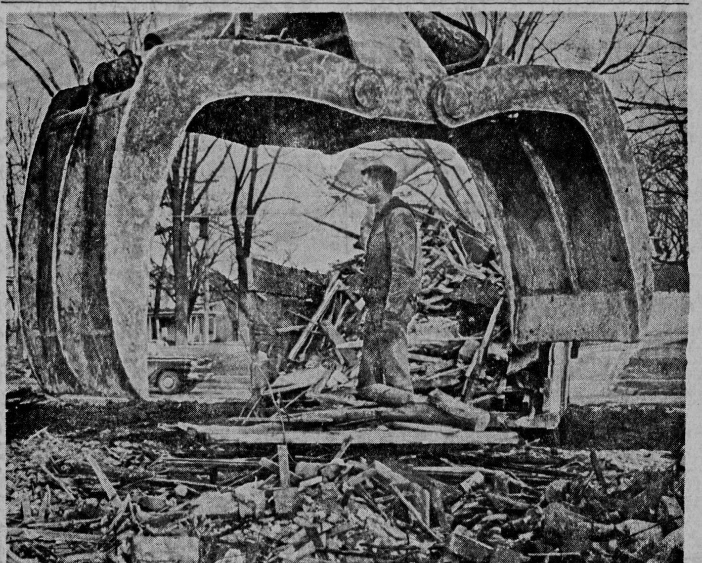
A DEMOLITION CRANE clears debris from a site on the 900 block of East Burlington Street where construction is soon to begin for a new Delta Gamma sorority house. The Delta Gammas
