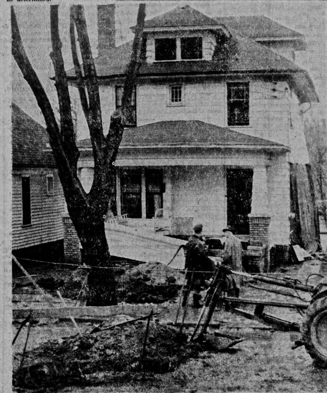
WITH THE PORCH RAILING DANGLING and one side bulging, the home of Mrs. John H. F. Miller and her daughters, Elsie and Helen, still stands after a gas explosion Sunday night. What set off the explosion, which injured Miss Elsie Miller, SUI statistician, has not been determined. The source of the gas leak was found near the hole in the lower left corner of the picture. The Miller home is at 1029 E. Market St.
