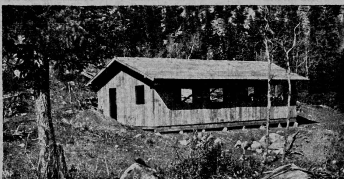
SHOP BUILDING of the Rocky Mountain Hydraulic laboratory near Allenspark, Colo., was partially completed when this photo was made in mid-August last year.
